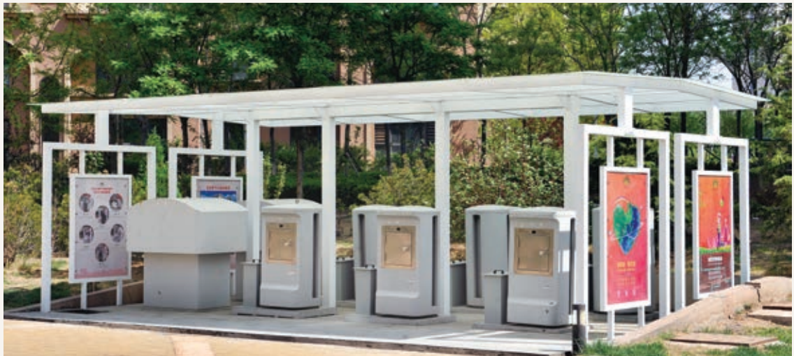
Pneumatic Waste Conveyance System (PWCS) collection bins at a residential development in the SSTEC Photo: Eco-city Administrative Committee
