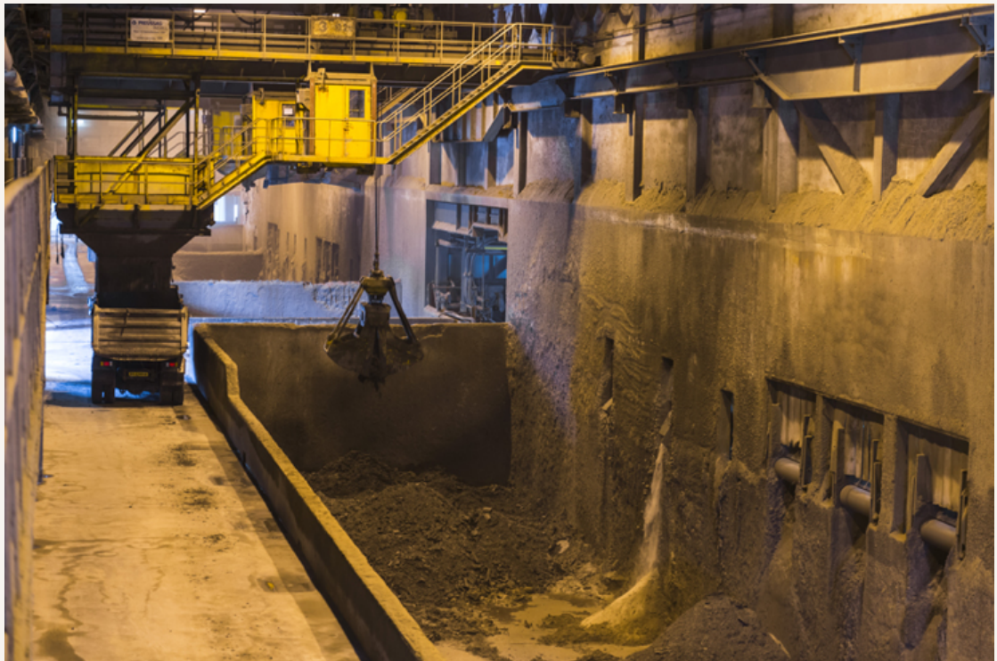
IBA pit at Tuas South Incineration Plant. NEA is studying the use of IBA for non-structural construction purposes.
